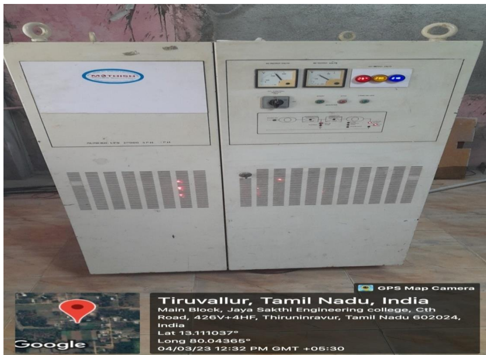
Uninterrupted Power Supply (UPS)
