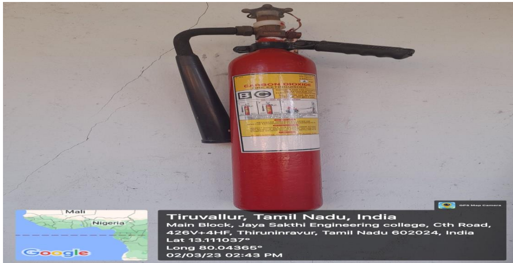
Fire extinguisher are installed for the safety of the College
